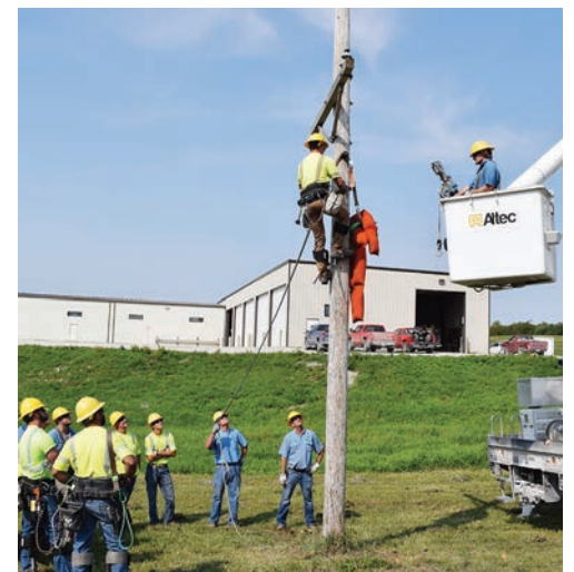
Lineman Mike Auten is evaluated for pole top rescue techniques as fellow linemen look on. In the bucket is Lineman Chad Berrey. The training is provided by the Iowa Association of Electric Cooperatives.
