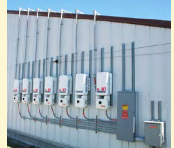
▲ A set of string inverters
